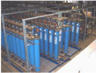
Figure 1: HYDRAcap Installation at Seedy Mill WTW
